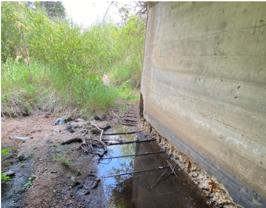
Picture 3 – CBC Bottom Slab Deterioration
