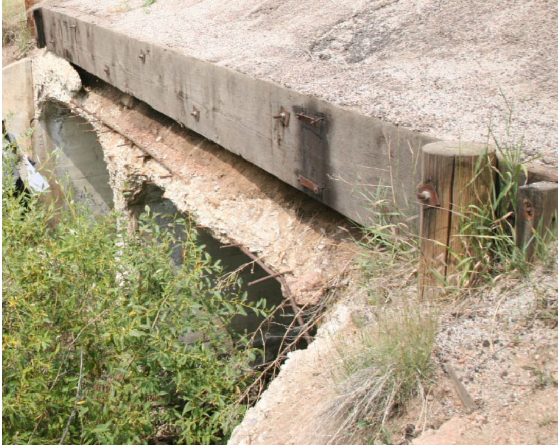
Picture 1 – South Headwall Deterioration
