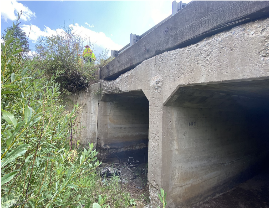
Picture 2 – North Headwall Deterioration
